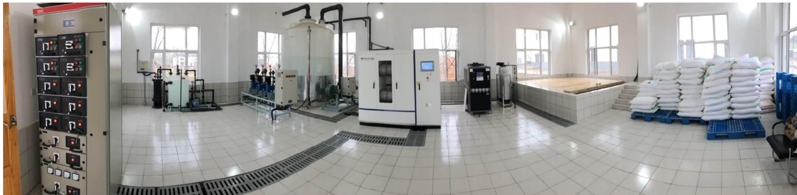
Juxian Water Plant
