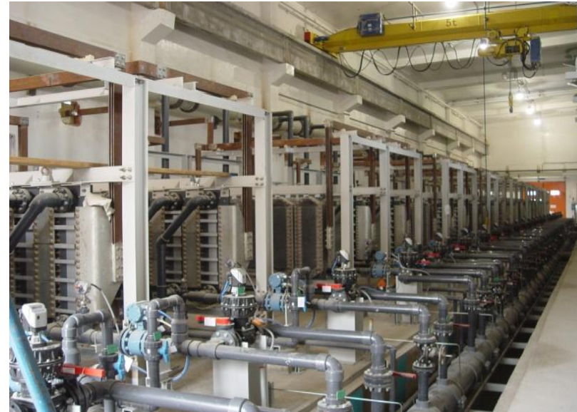
Hongyanhe Nuclear Power Plant
