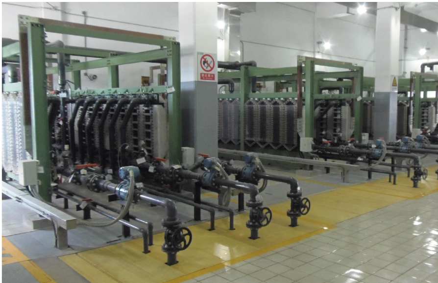
Sanmen Nuclear Power Plant
